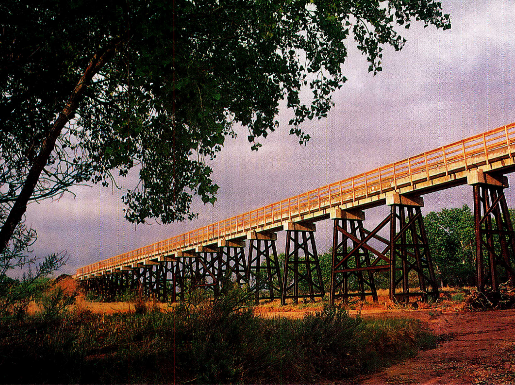
High and dry. The longest span on the Trailway, the concrete Los Lingos Bridge once ensured a safe creek-crossing for trains on the Fort Worth and Denver Railway.
