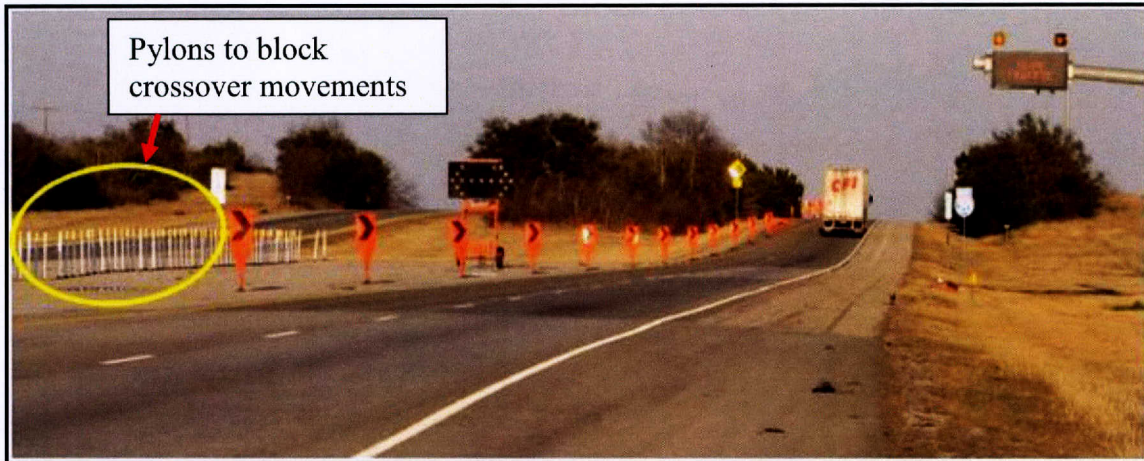
Figure 12. Pylons Blocking Crossover Movements, Rural Highway, IH 20, Ranger Hill, Texas.
