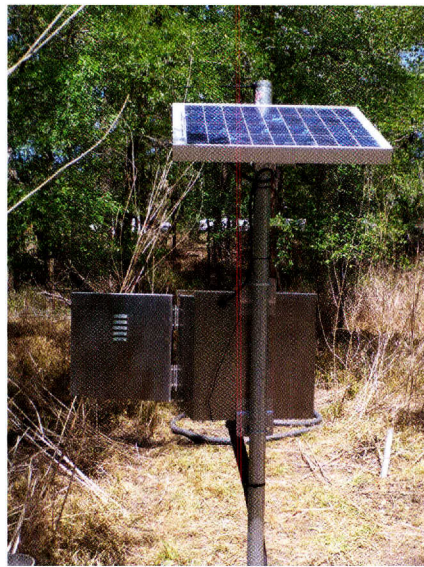
Continuous Water Quality Monitoring Station control and power center in the Guadalupe River Basin - Photo by GBRA
