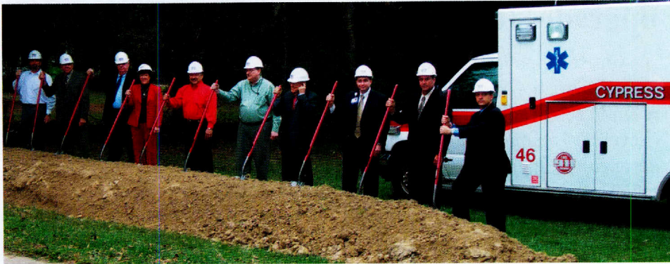
In January of 2009, the Cypress Creek EMS complex will include administrative offices, an education center, a communications center and an EMS station. CCEMS Board of Directors, from L to R: Greg Marwill, president; Jim Cravens, president-elect; Dave King, secretary; Karen Plummer, corresponding secretary; Ruben Gonzales, Jr., director; Dennis Schmidt, volunteer representative; Bill Carey, director; Drew Kahn, director; Brad England, CCEMS executive director; Dr. Levon Vartanian, CCEMS medical director.
