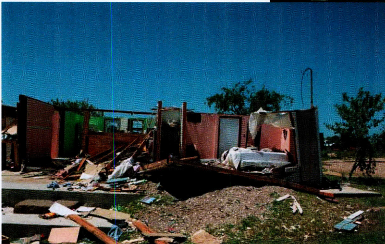
The tornado that hit south of Eagle Pass on April 24 killed seven people and sent dozens to Fort Duncan Medical Center. Winds also damaged hundreds of structures.
