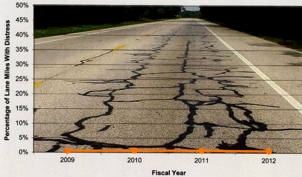
ACP Block Cracking (rated), FY 2009-2012
