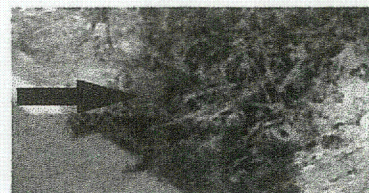
Broken, leaking sprinkler head
