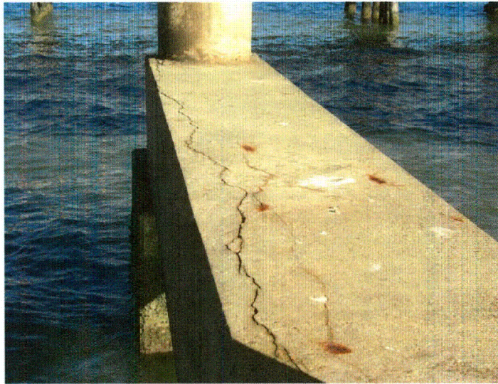
Figure 6.4: Cracking of Tie Beam
