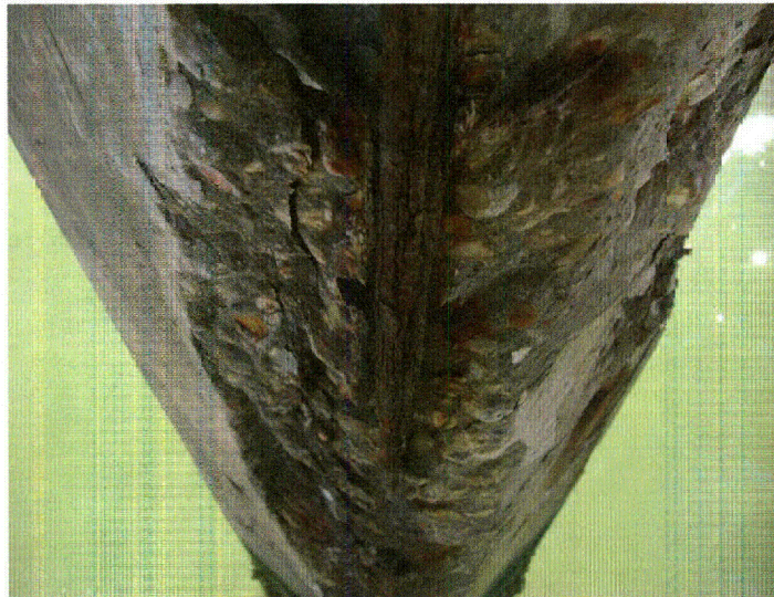
Figure 5.5: Corrosion of Precast Concrete Piling
