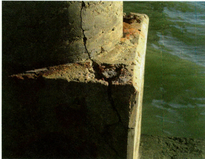
Figure 6.2: Corrosion of Tie Beam and Column
