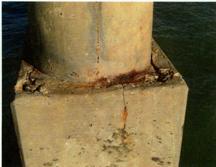
Figure 6.3: Cracking of Tie Beam and Column
