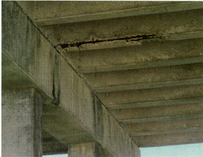
Figure 6.6: Corrosion of Concrete Slab and Girder Span
