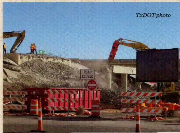
Crews demolished the southbound Quaker Avenue/TTU Parkway bridge on northwest Loop 289 in December 2012 to make room for the new bridges that also span over Erskine Street. The $26.9 million project widened Loop 289 from four to six lanes.
