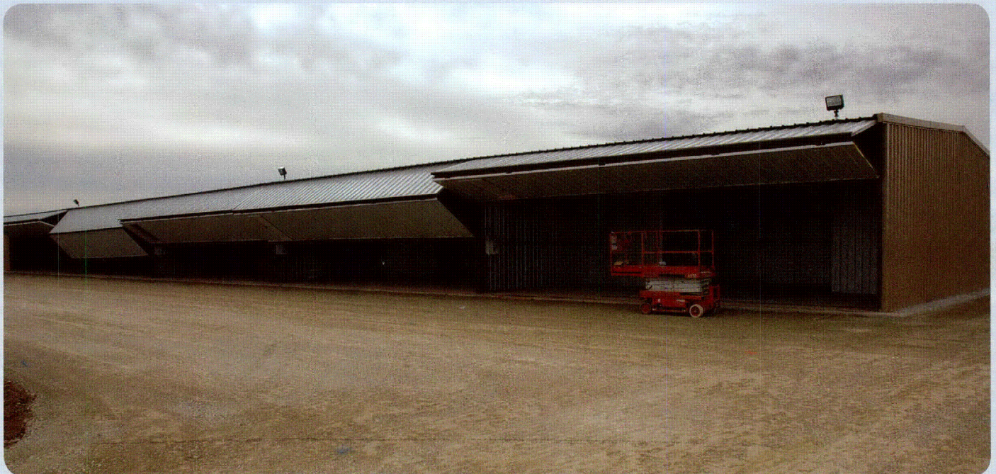
A 10-unit T-hangar and new hangar access taxiway under construction at the Goldthwaite Municipal Airport.
