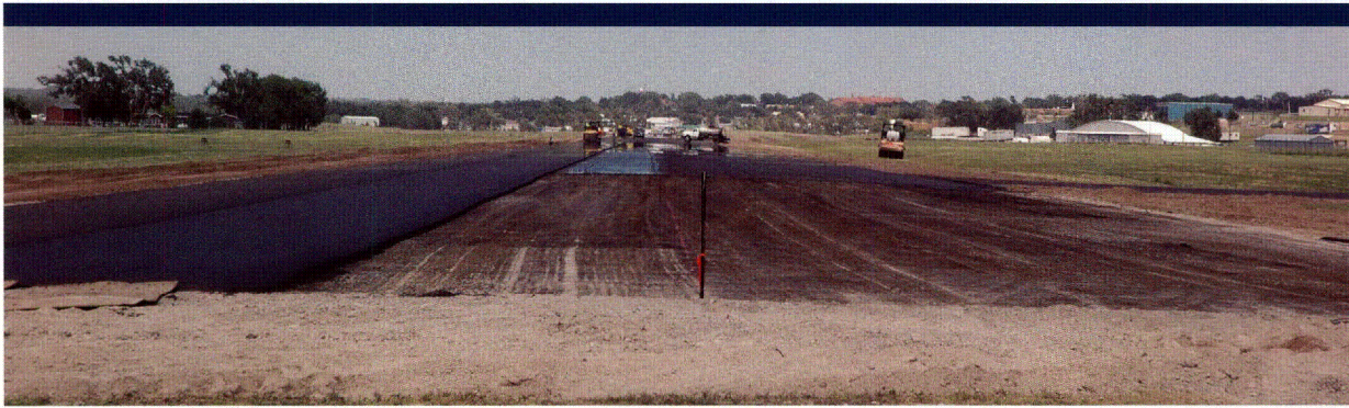
Construction crews put the finishing touches on runway 4/22 at Hemphill County Airport in Canadian.
