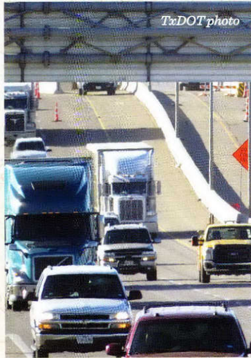
Work has begun on I-40 in Amarillo to completely rebuild the bridges located at the Ross Osage Drive and Arthur Avenue intersections.
