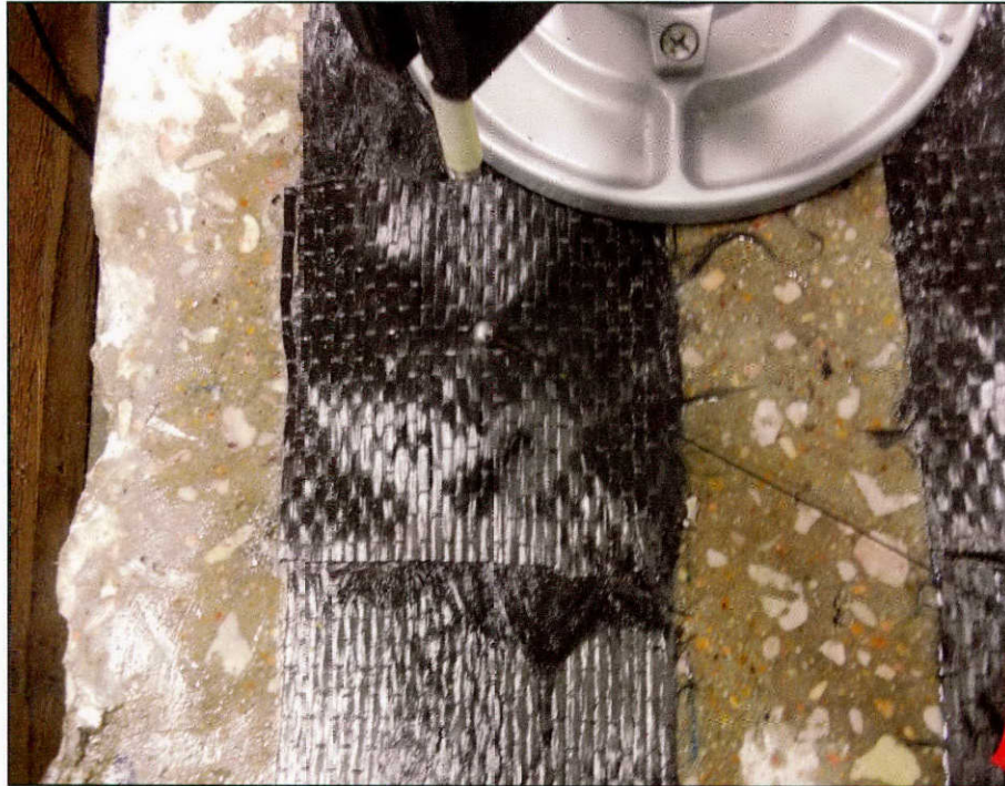
Figure 7-9: Anchor defect detection using the sounding method
