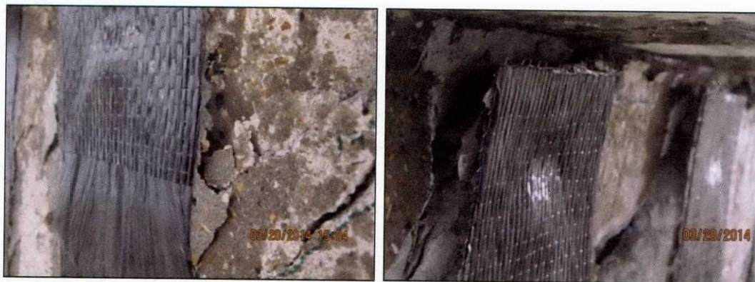
Figure 3-26: Concrete crushing behind anchors (24-3-8-2)
