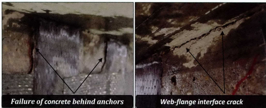
Figure 3-28: Flange-web crack interface (24-3-8-3)
