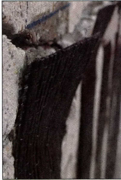
Figure 5-27: CFRP anchor post-failure
