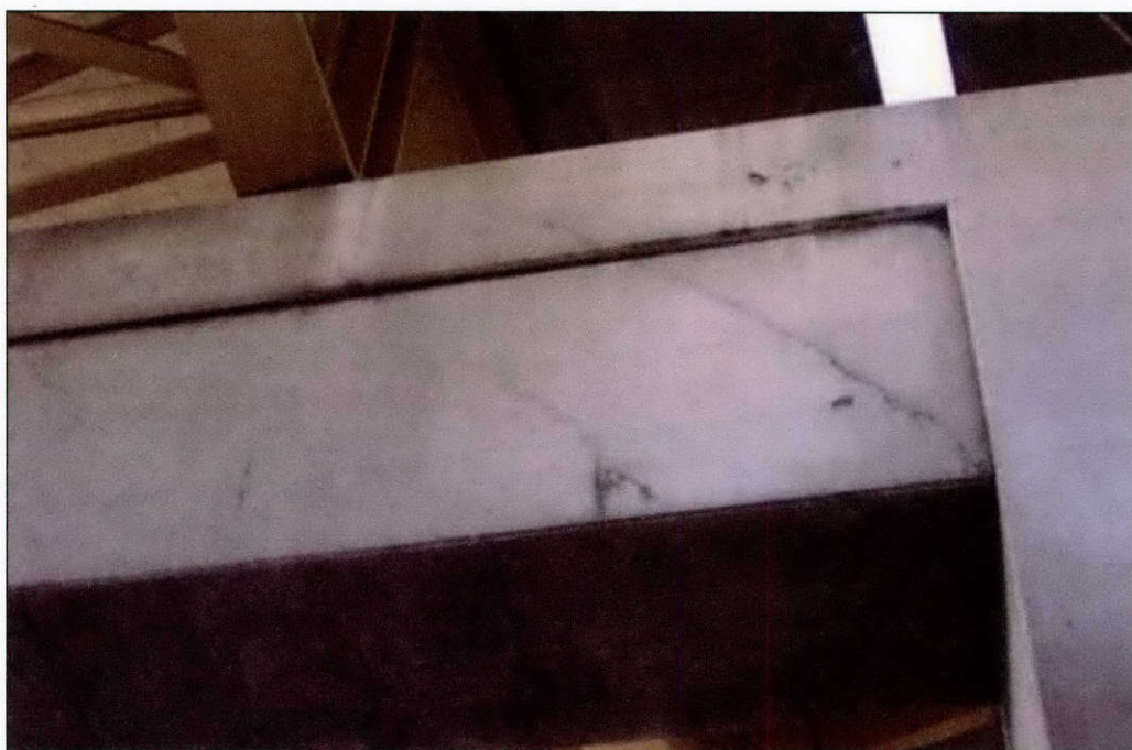
Figure 5-1: Shear crack in pile cap girder
