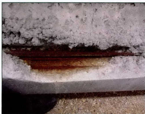
(a) Before repair
